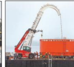
Above, cable is unraveled from a large spool, located topside at mid-ship, before being fed off the stern of the barge and onto the seabed.
